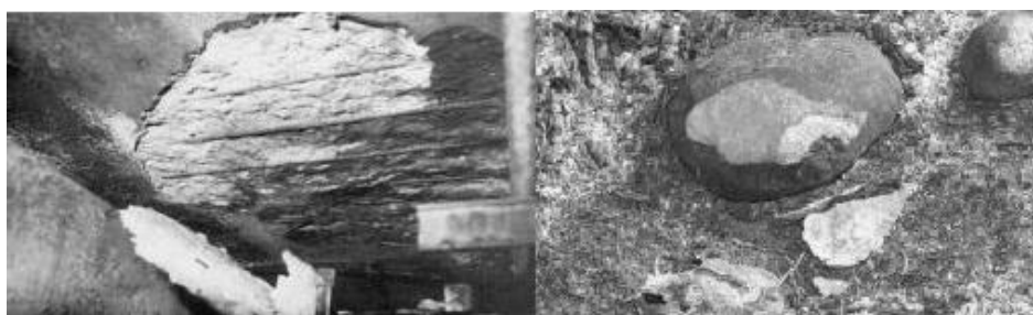
Figure 1 – Spalling: (a) in reinforced concrete slab and (b) in rock Source: [9].
