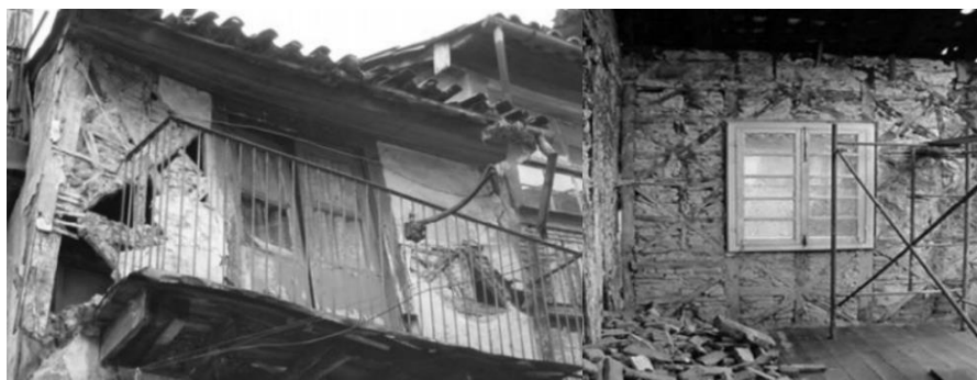
Figure 4 - Degraded masonry walls Source: [1].
